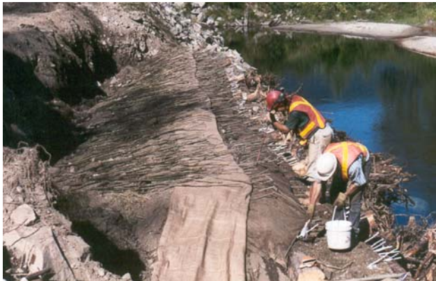
Bio-engineering techniques (willow shoot layering) being used to rehabilitate a stream bank near Edgewood, B.C.
