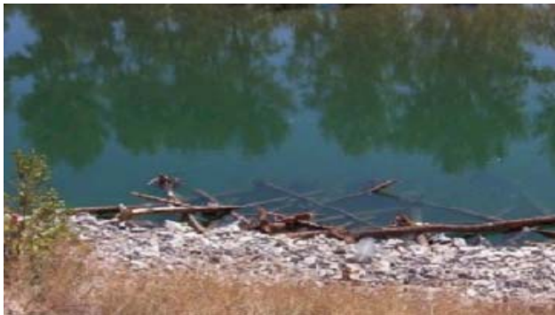
Habitat compensation structure (visible portion) on Elk River at Elko, BC. Would this structure be acceptable on the Slocan?
